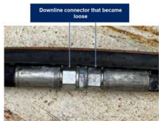
BSP fitting which came loose
