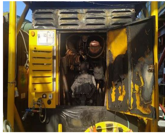
Damage to interior of compressor
