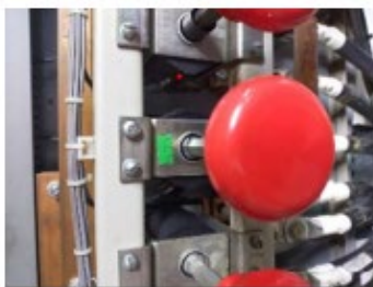
Battery disconnect switch
