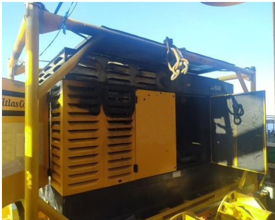
Compressor on deck
