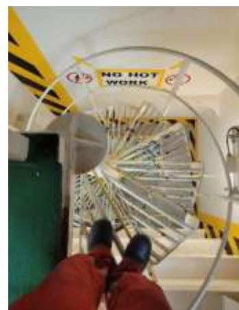
Spiral ladder which would not have allowed passage of a stretcher
