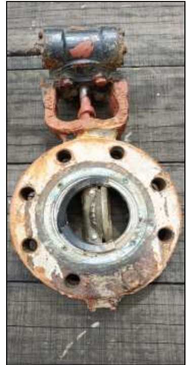
Showing damage on valve surface and seal
