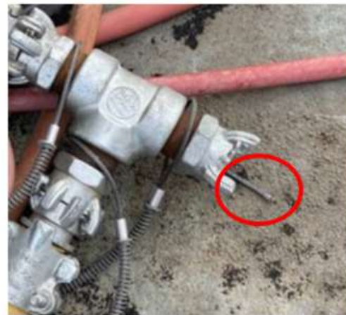
Figure 2 - Broken whip check from the incident.
