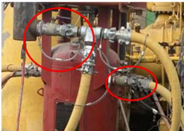
Figure 1 – Temporarily installed air dryer with bull hose connections. Original whip check position (Left Circle) and the location of the injured persons hand placement on the air supply valve (Right Circle).
