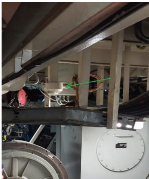
Smoke detector over the affected Shaft Generator
