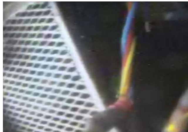
Subsea camera still of twisted umbilical
