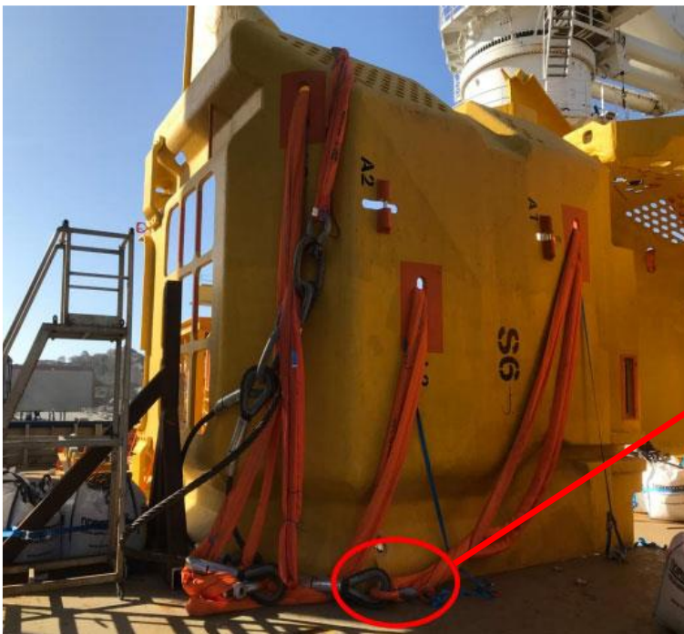
Lift rigging fell from flat top section of hatch cover
