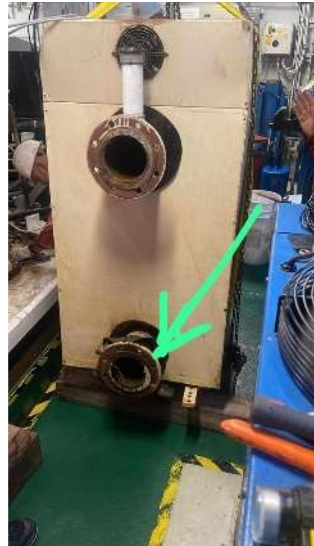
Location of the hole, inaccessible for visual inspection. Picture shows the back part of the unit mounted against a wall.
