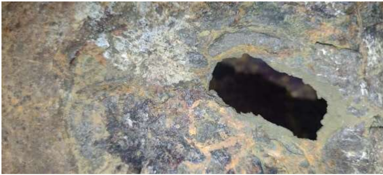
The hole at 6 o'clock in the water intake.
