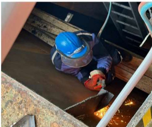
Welder’s initial position without any fall protection
