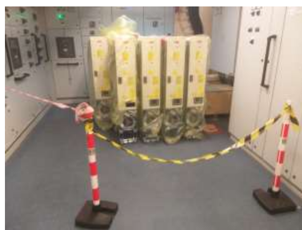
Showing wheeled control cabinets each weighing 130kg
