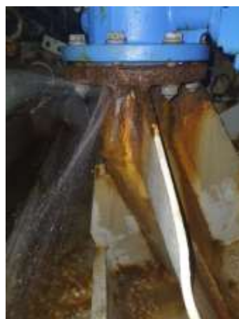
Deteriorated condition of sea suction pipe leading to leakage
