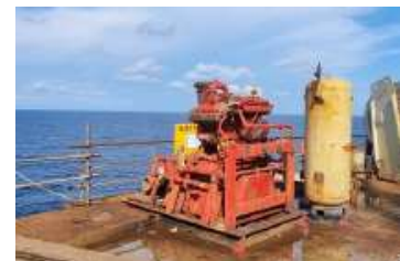
A similar fire water pump skid and Nitrogen tank set up
