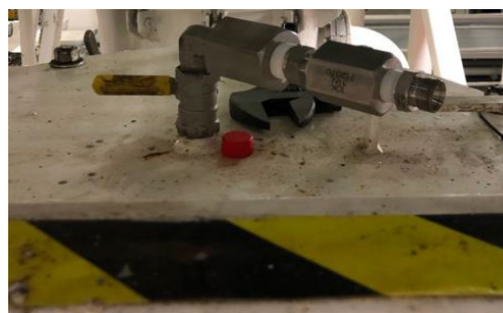
Vent valve on top of unit
