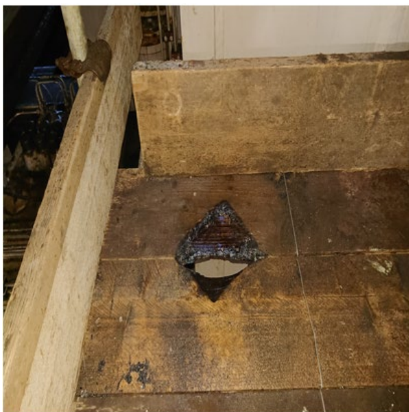
Damaged scaffold board
