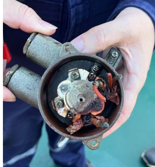
Electrical switch showing clear sign of water ingress
