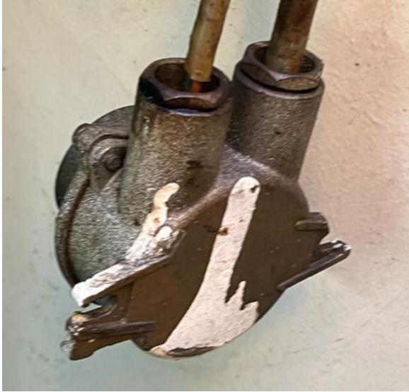
Appearance of electrical switch to visitor
