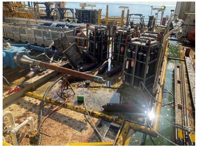
Where the rupture occurred
