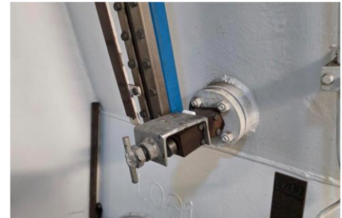
Showing a home-made clamp which ought not have been there
