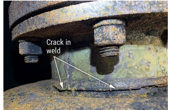
Crack in weld below the upper (outlet) flange of the starboard muffler
