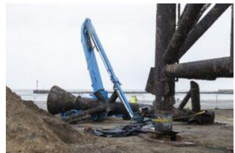
The skirt pile gave way and struck a mobile elevating work platform
