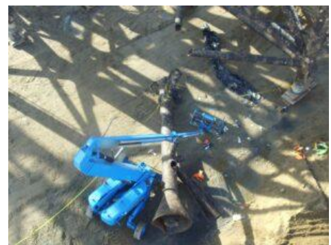
Where the workers fell
